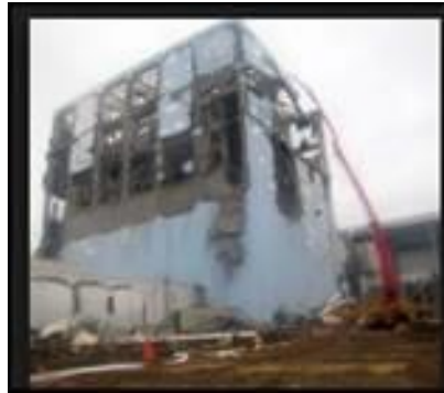
Fukushima Daiichi, Unit 4- Hose adding water to pool, reactor building is a shell after explosion
